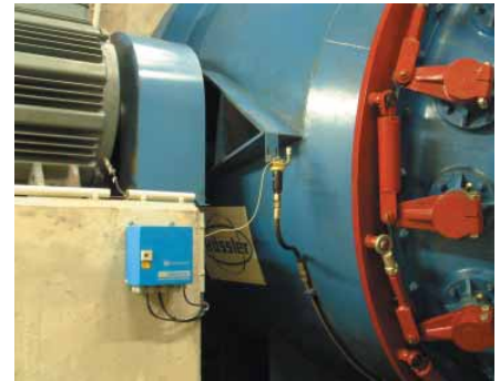
VIBNODE® online monitoring
