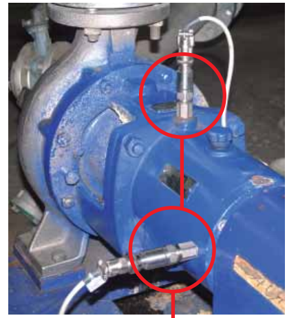
Vibration sensors in the area of the pump shaft bearing
