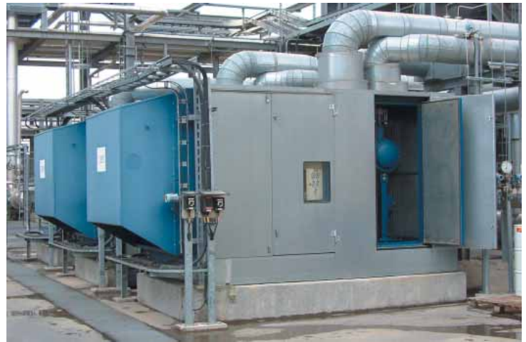
Screw compressor in a plastics plant
